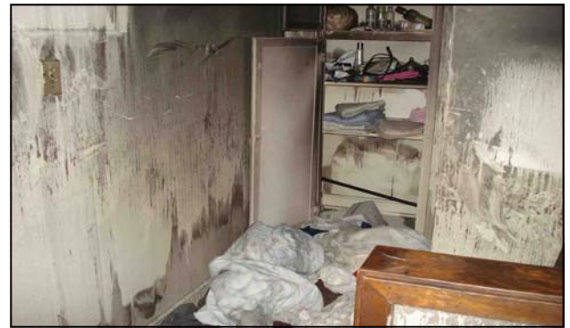
Fire, Smoke, and Odor Damage Affects Structure and Contents Inside Housing Authority Unit.
