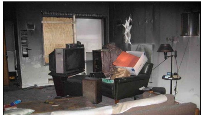
Fire and Smoke Damage Inside Housing Authority Unit.
